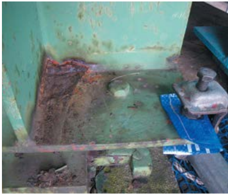
(a) Local corrosion of plate girder
