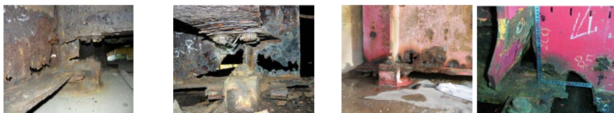
Fig. 1 Corroded plate girder around support
